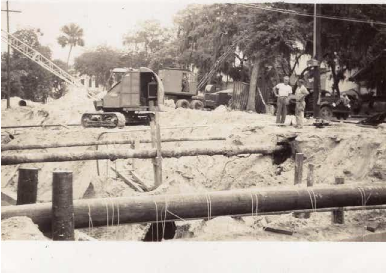
In the early 1900s, a canal ran along Bay Street from Nova Road to the Halifax River to drain water. In the mid-1900s the city filled in the canal and added drainage pipes. Photo provided by Bonnie Decker Tippets
