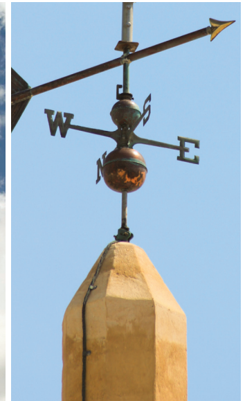
Figure 13. A new lightning rod was also installed. PHOTOGRAPHED BY RANDY JAYE ON JUNE 27, 2016.
