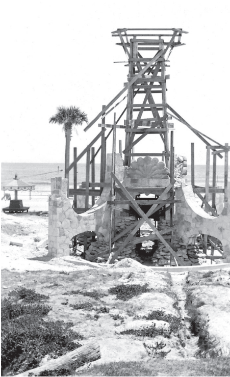
Figure 4. Under construction, circa 1936. The base and French buttresses are complete, with scaffolding in place to build the body of the structure. PHOTO COURTESY OF THE HALIFAX HISTORICAL MUSEUM.
