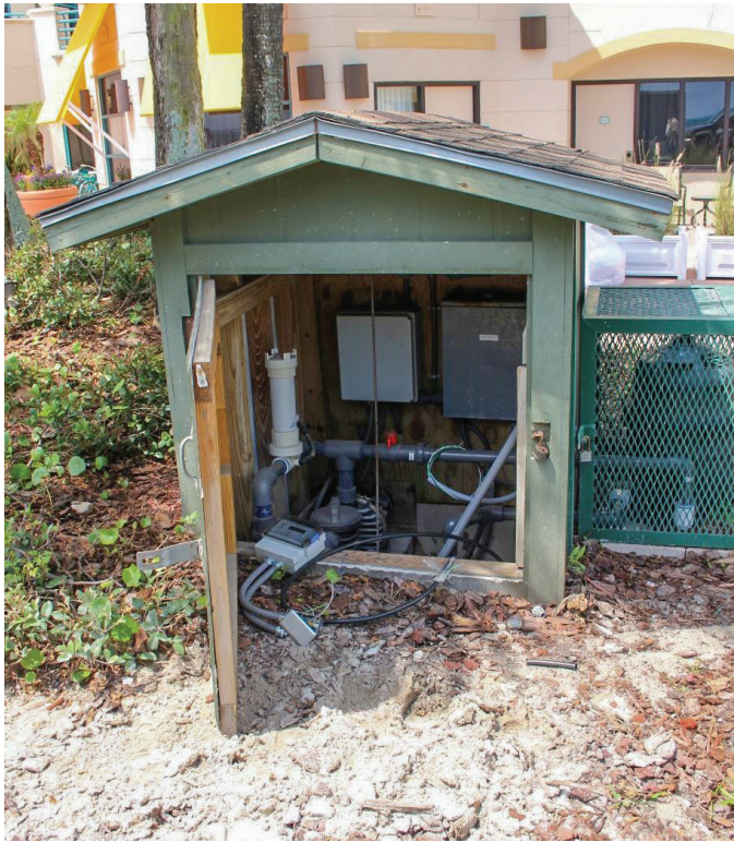
Figure 15. Clock tower pump house. New model MCCE Master Clock Controller being installed. PHOTOGRAPHED BY RANDY JAYE ON JUNE 10, 2016.
